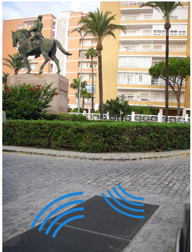
Fibrelite FM45 covers installed allowing RF signals to pass freely through. Photo credit: Aguas de Cádiz
