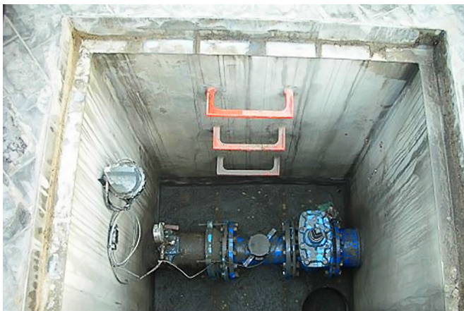
Automatic monitoring system located beneath metal cover which blocked signal. Photo credit: Aguas de Cádiz
