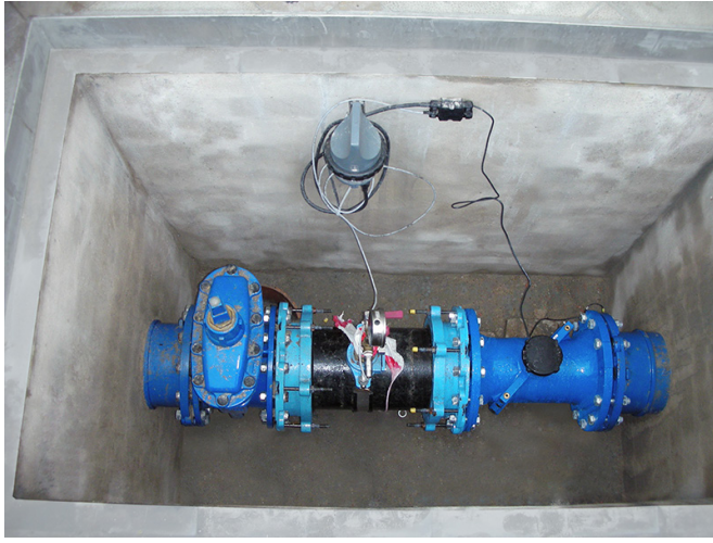
Underground water monitoring system. Photo credit: Aguas de Cádiz
