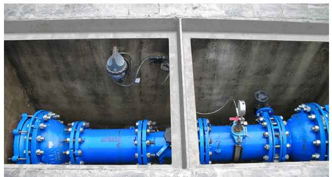
Fibrelite trench covers fitted into existing frames, preventing expensive breakouts and time for concrete to set. Photo credit: Aguas de Cádiz
