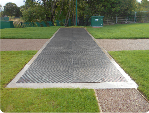
The Fibrelite B125 (12.5 tonne) load rated medium duty trench access covers installed
