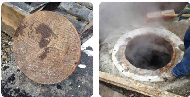
Large cast iron covers are both very heavy and extremely hot when exposed to steam within the manhole
