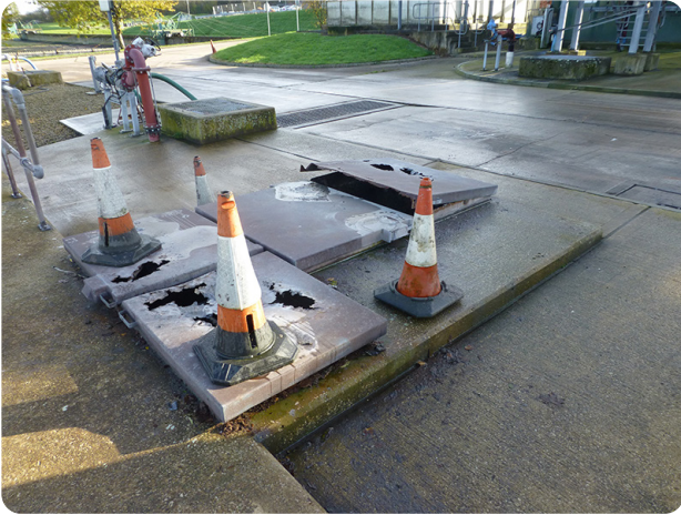
The previously installed dangerous and corroded metal covers
