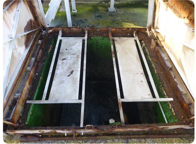
The old heavy mechanical steel covers were replaced with the Fibrelite lightweight alternative
