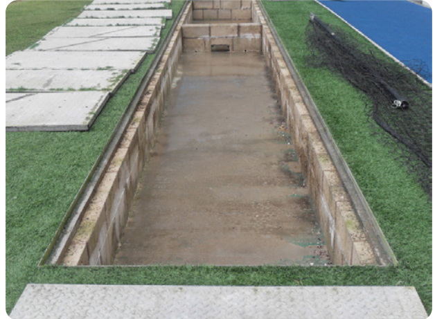
A camera pit to be covered by Fibrelite composite trench covers
