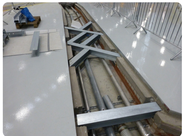
Fibrelite covers needed to be manufactured to work with pre-installed steel supports
