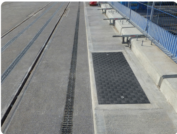
Bespoke trench covers for trackside gear
