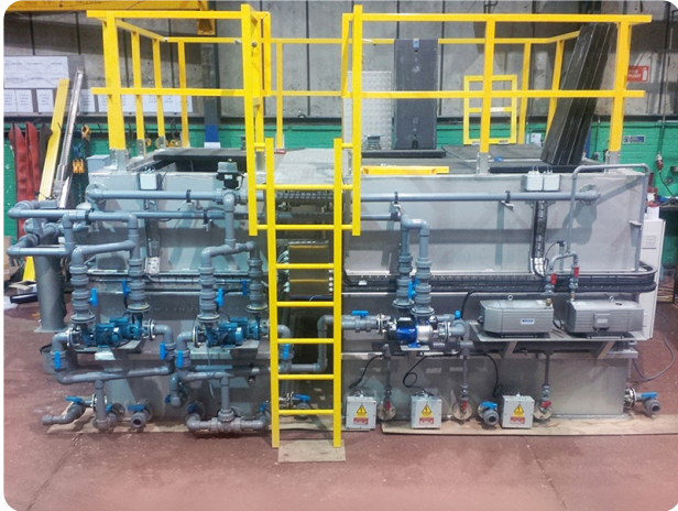
The specialist waste water treatment system at this plant
